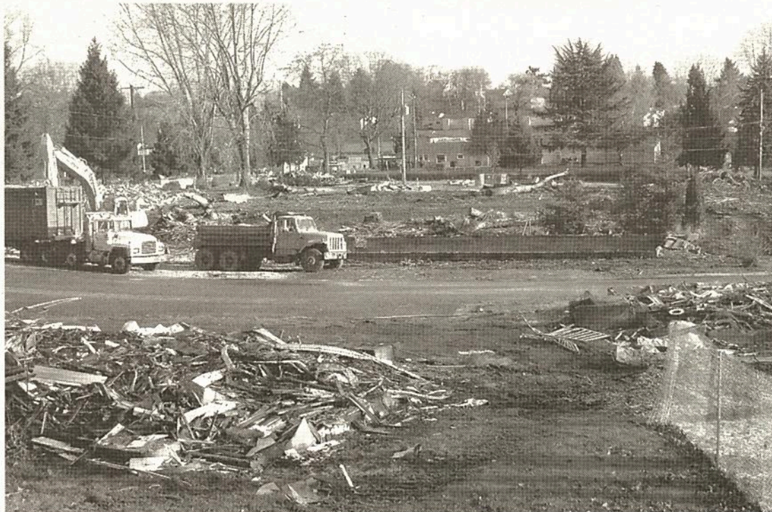
DEMOLITION AT RAINIER VISTA RESUMED AFTER A SETTLEMENT WAS REACHED IN THE LAWSUIT AGAINST THE PROPERTY'S OWNER, THE SEATTLE HOUSING AUTHORITY. IN THE BACKGROUND, INTACT HOMES AWAIT THE WRECKING CREW. PHOTO BY SIGNE DRAKE.
